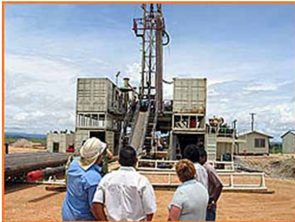
Natural Resources Minister Johnny Briceno (center) & BNE executives inspect Belize's first production oil well, Usher I.
