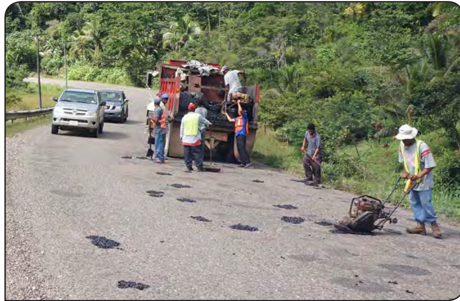
Short-term patching on portions of the Hummingbird Highway which will become unnecessary after complete resurfacing
